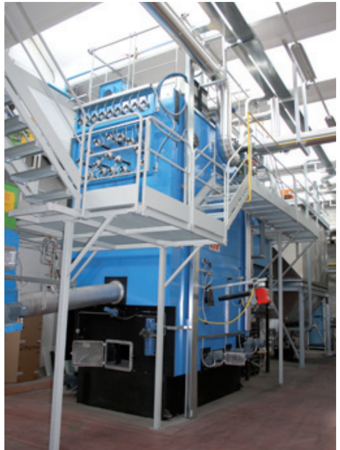
Figure 4 – Example of a woodchip boiler for heating greenhouses.
