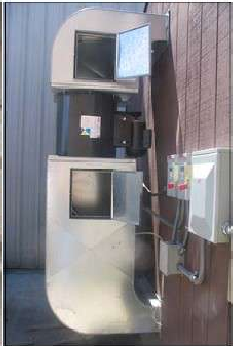
Figure 9: Duct work and access doors housing heating elements and fan
